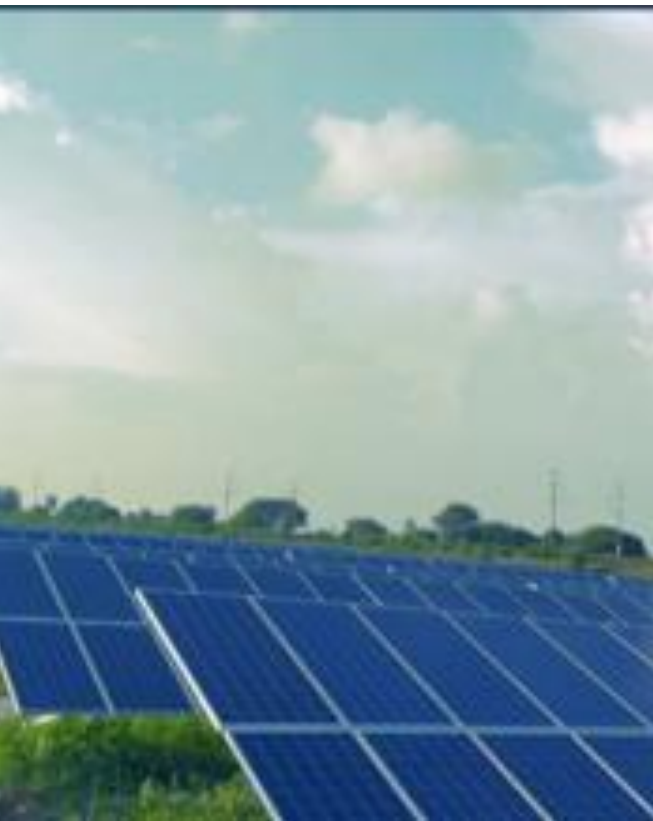
2.6 MW Dc Solar Plant
